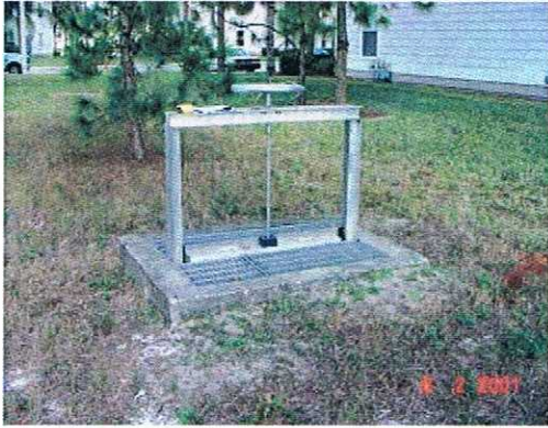
Figure 1: Example of Operable DCS community outfall pipe
