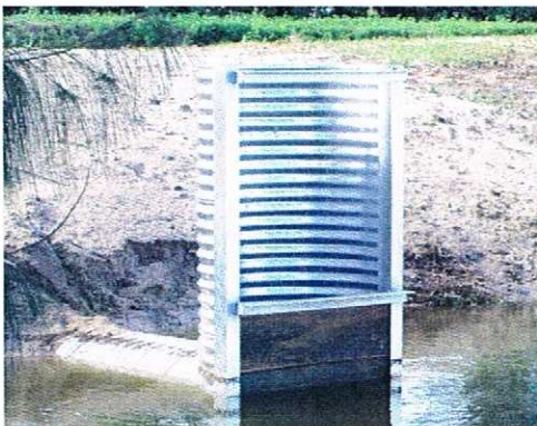
Figure 3: Example of adjustable boards on a Flash Board Operable DCS
