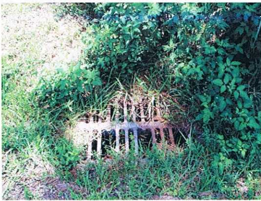
Figure 6: Example of vegetation obstructing flow in drain
