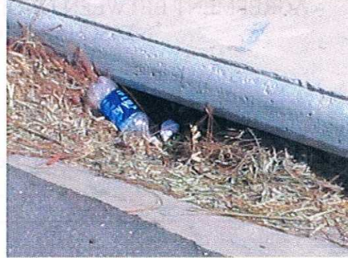
Figure 5: Example of vegetation and trash obstructing flow in drain
